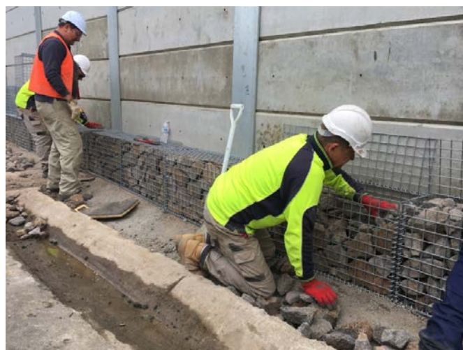
Work begins on the Gabian rock wall on the Great Ocean Road.
